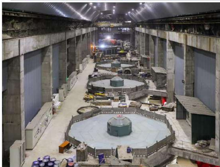
Machine Hall of Punatsangchhu-II HEP, Bhutan
